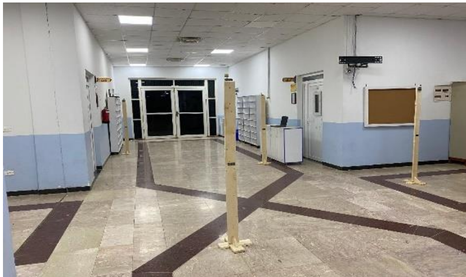
Figure 2 The installed anchor nodes in the real environment
